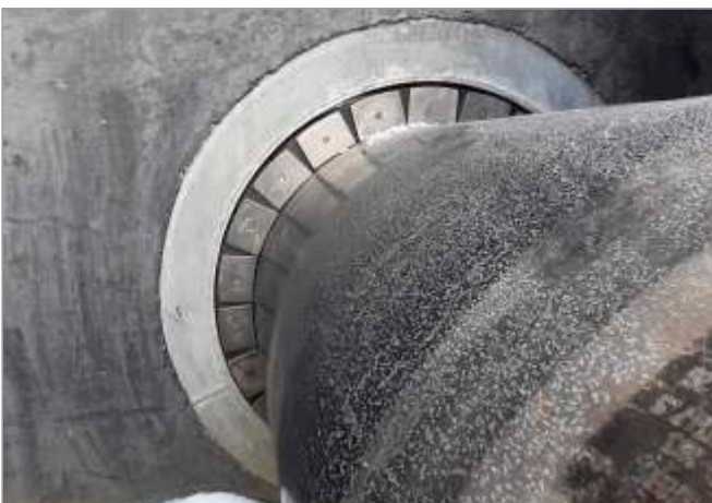
36 Sewer pipes 600 mm diameter
