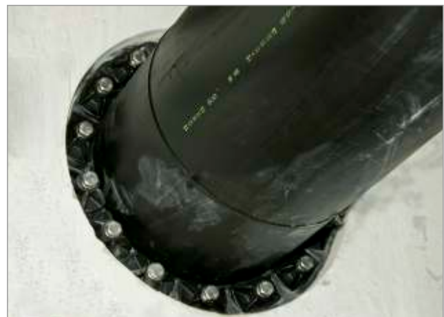
Water pipelines 250 mm diameter
